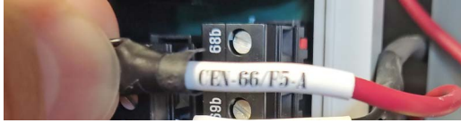
Wire 66 taped off and not used
